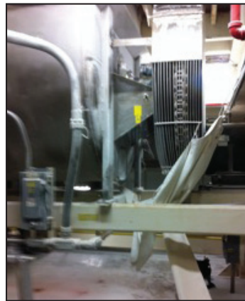
A bag catches pancake mix leaking from a mixer due to failed shaft seals, while additional leaking mix piles up on the ground.
